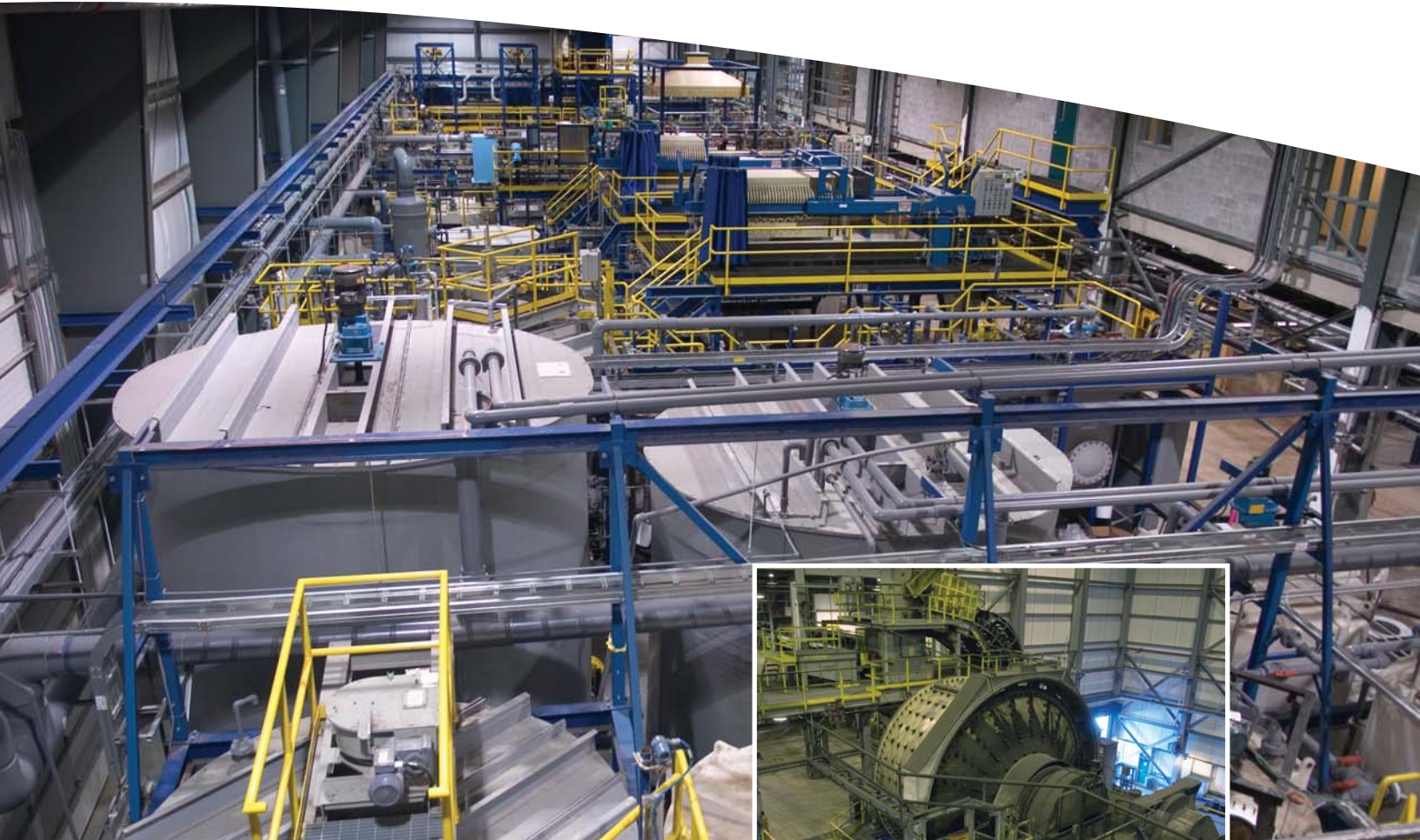
Hydrometallurgical Demonstration Plant interior, Argentina, Newfoundland
